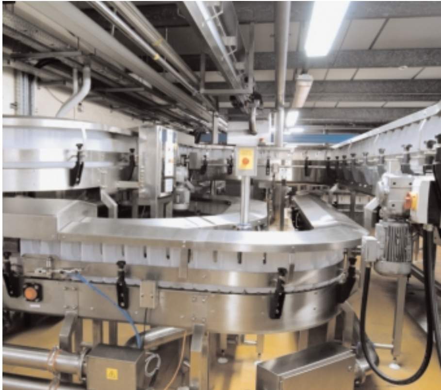
World-class milk bottle manufacturing equipment at the in-plant dairy operation at Oakthorpe in the United Kingdom
